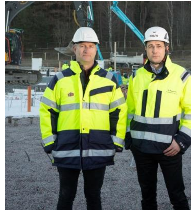
Patrik Ahlberg, CEO of Arboga Bostäder and Fredrik Leo, CEO of ByggPartner, in place at the foundation of Åspegelns elderly housing, Arboga, 2019.
